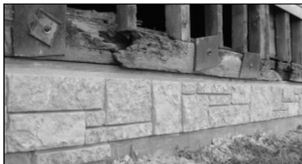
New masonry contrasts with rotten sill that will be replaced in the coming months.
